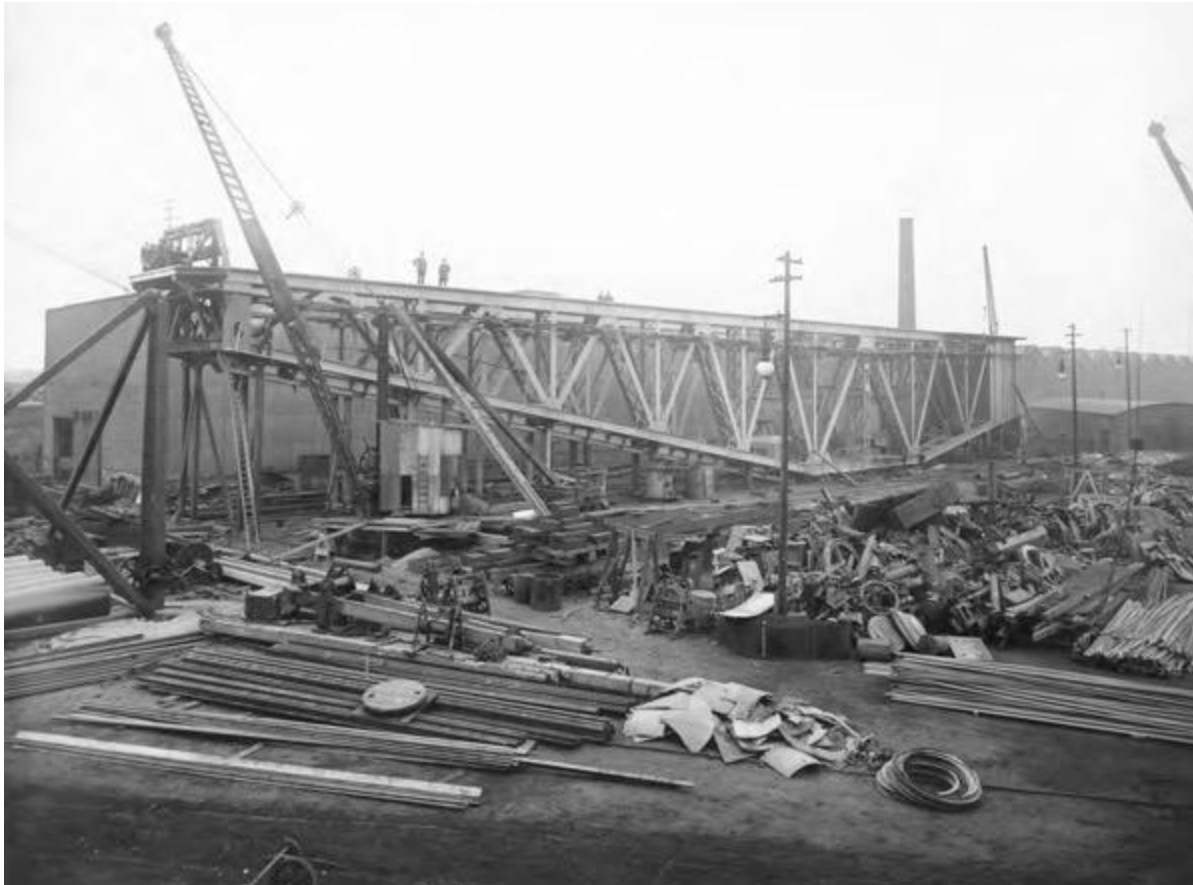
Figure 4: The jib of the Sasebo Giant Cantilever Crane, at Arrol's Parkhead Works prior to being dismantled and sent to Kyushu, Japan, c.1911. (SC555106, ©Courtesy of HES, Sir William Arrol Collection)
